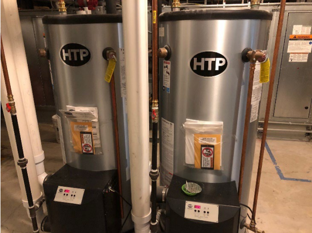
Hot Water Heaters
