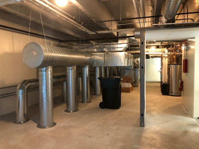
Mezzanine Level Mechanical Room
