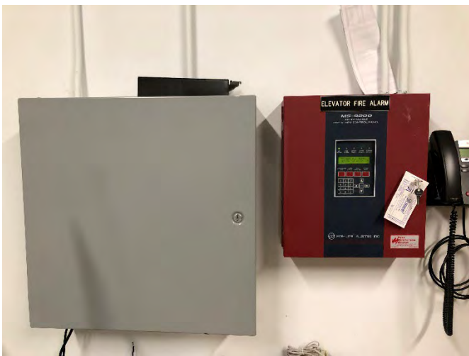
Fire System Panel
