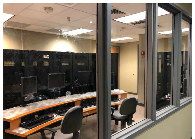
Secured Data Center
