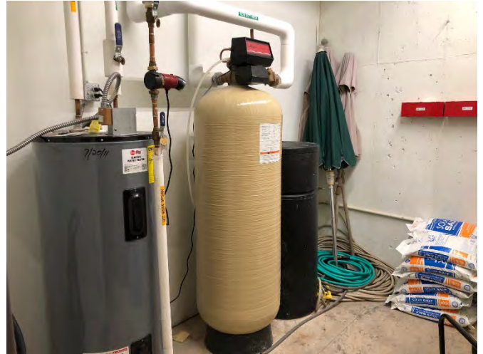
Water Softening System
