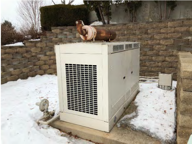
81 Kw Spectrum Brand Generator
