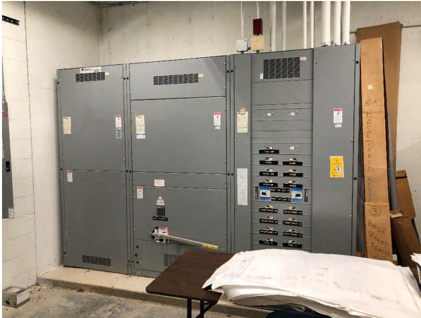
Main Electrical Switch Panels
