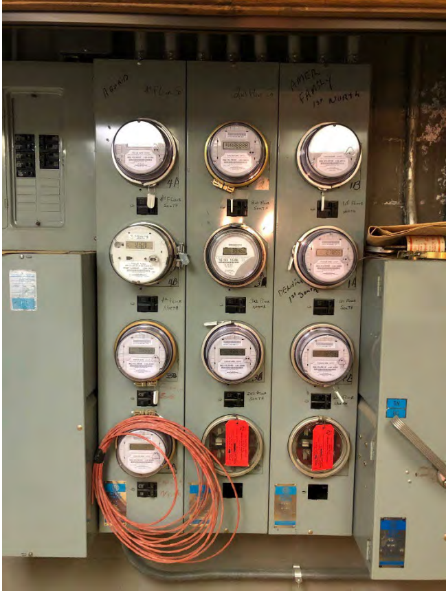
Electric meters for suite metering of overhead lights & convenience outlets.
