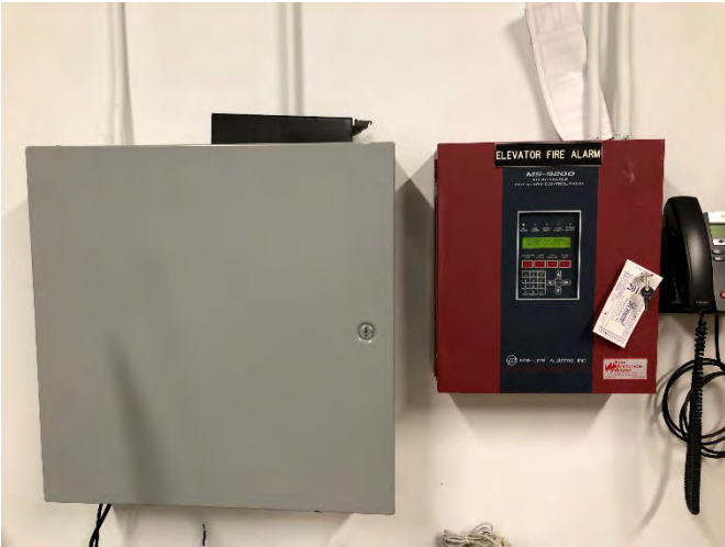
Fire System Panel
