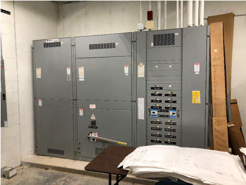
Main Electrical Switch Panels
