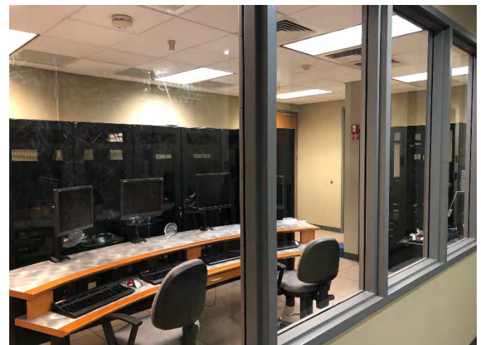
Secured Data Center
