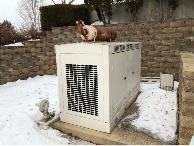
81 Kw Spectrum Brand Generator
