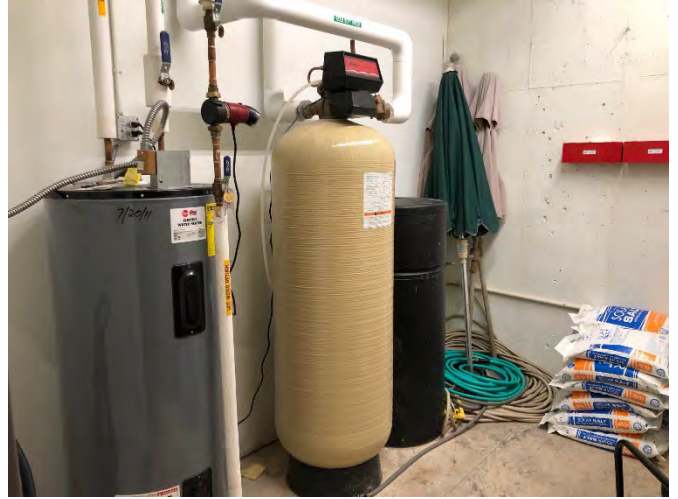
Water Softening System
